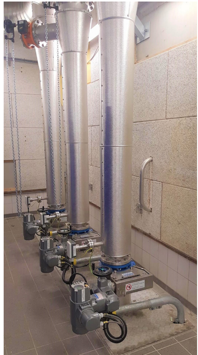
Precision flow control was an essential part of the installation
